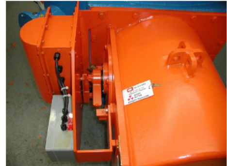
Figure 12: electric shutter mechanism. (note also the padlock key with its emergency information tag)
